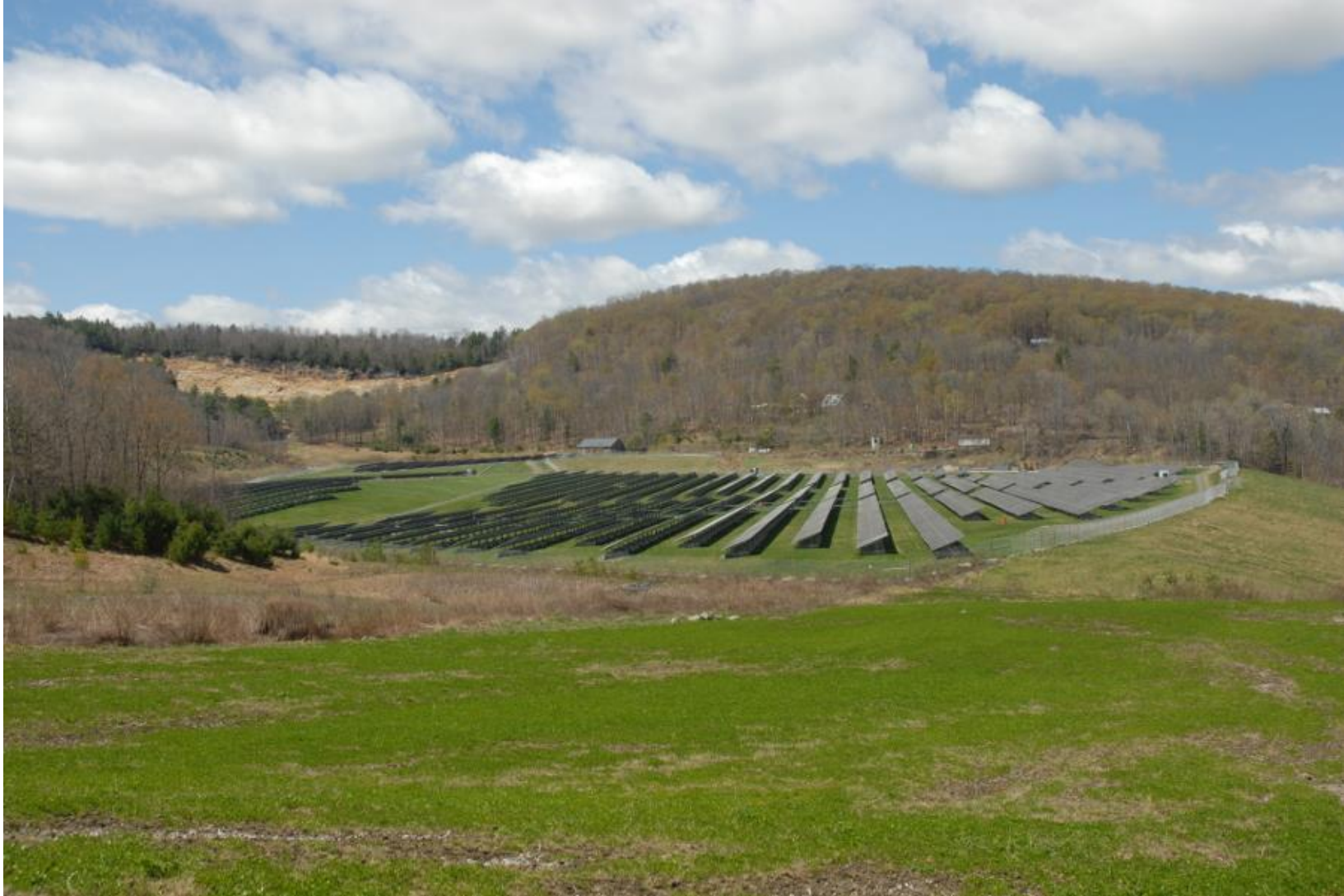
39. Solar Electric Panel Array looking southwest (Milestone Heritage Consulting, May 2021).
