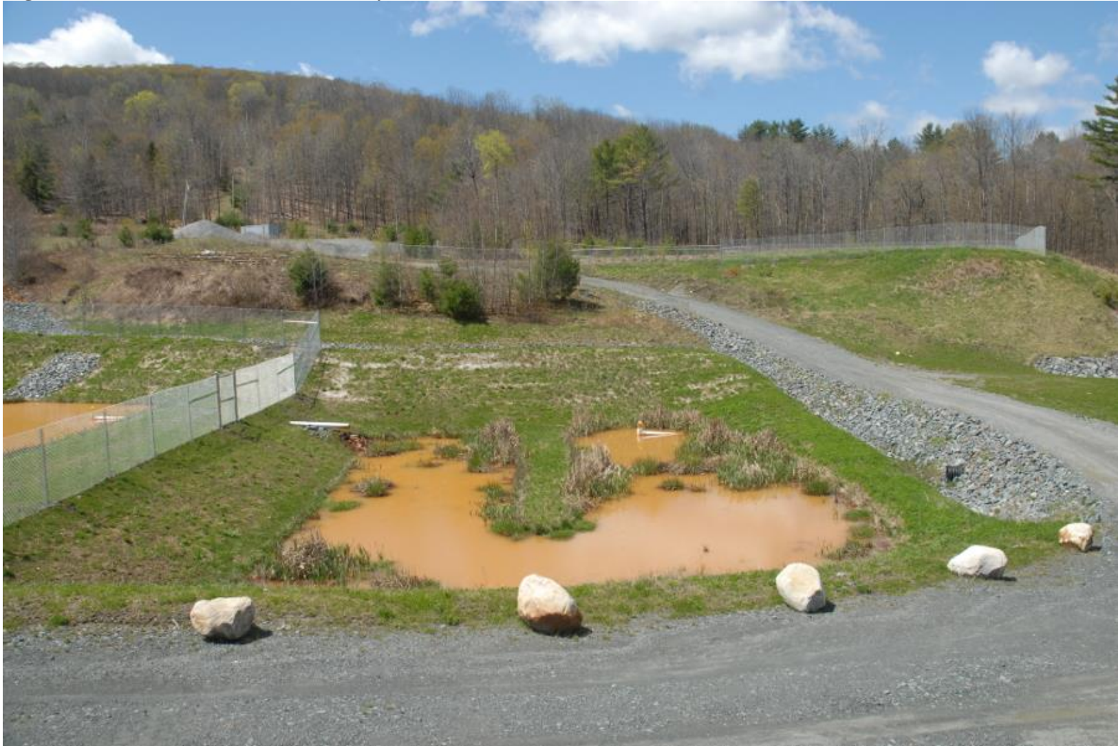
28. Passive Treatment System looking west showing initial wetland (Milestone Heritage Consulting, May 2021).
