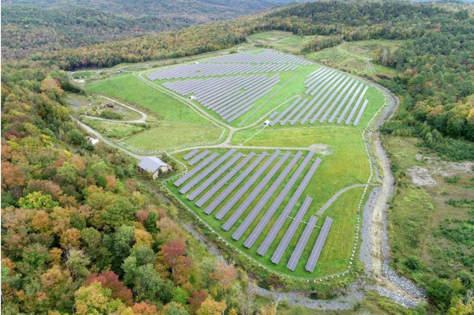
32. Aerial view of Solar Electric Panel Array looking northeast (Doucet Survey, September 2021).
