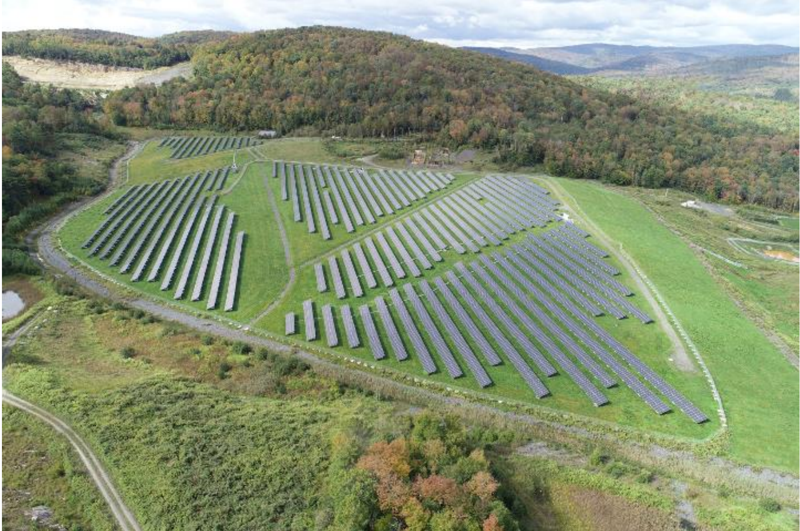
34. Aerial view of Solar Electric Panel Array looking west (Doucet Survey, September 2021).
